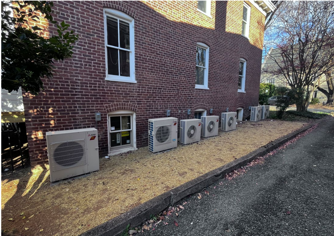
Mechanical units at side yard, November 2024
